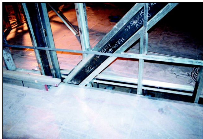
Figure 2: Gap where a structural wall extends to the slab.
